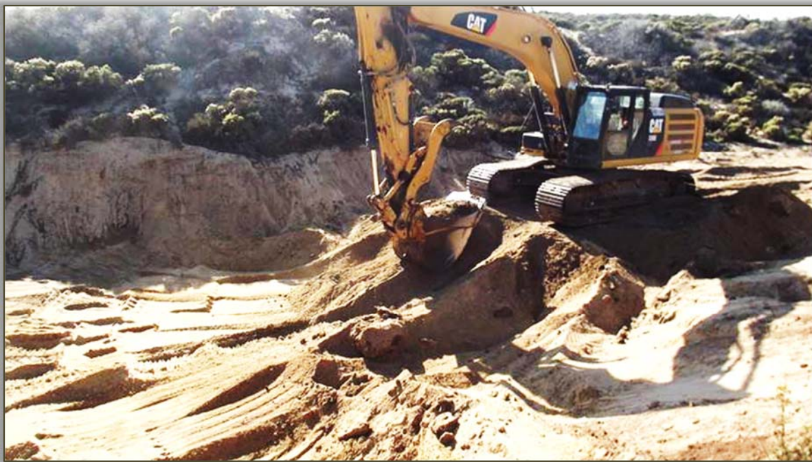
I6A PROs Site Excavation: diluent and sump material is excavated from the site prior to any pad or oil spray treatment.
