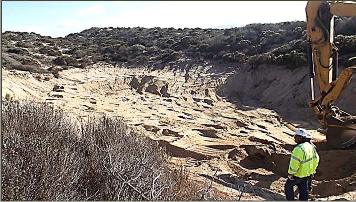
16A PROs Site Excavation: post excavation. Diluent and sump material is excavated to a depth of four feet or greater, samples are collected, and results are analyzed by Chevron, the RWQCB and the OEC prior to backfill approval.
