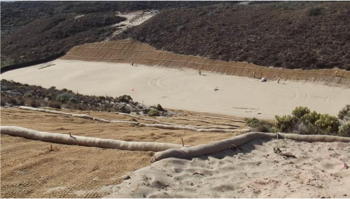
The M1 Valley: backfill along slopes has been completed, B&P measures are currently being installed including: placement of topsoil, jute-netting, sand fence, and application of hydroseed spray.
