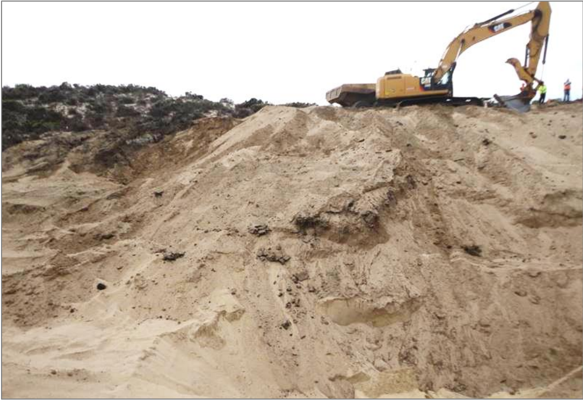
F7B PROs Site Excavation: diluent and sump material is excavated from the site prior to any pad or oil spray treatment.
