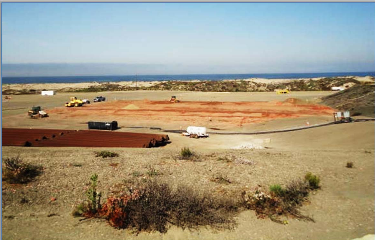
TB8 Basin: currently backfilled and are being capped with red rock and asphalt to eliminate exposure and storm water runoff concerns.
