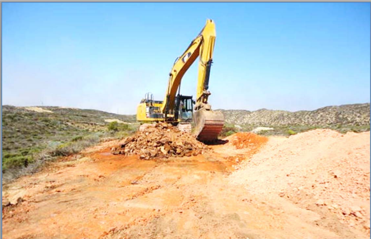
M14 Road Removal (as part of the final Phase II PROs activities).
