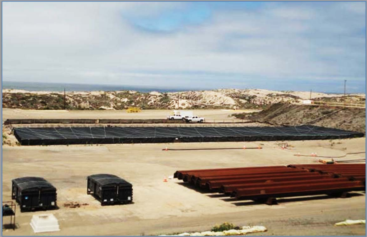
TB8 Basins: Chevron continues to decommission the TB8 Basins (old view of tarp-covered basins in background). These basins use to contain contaminated water and were responsible for continued potential exposure risks to wildlife. Both basins are now currently backfilled with contaminated material (excavated from the PROS Sites).
